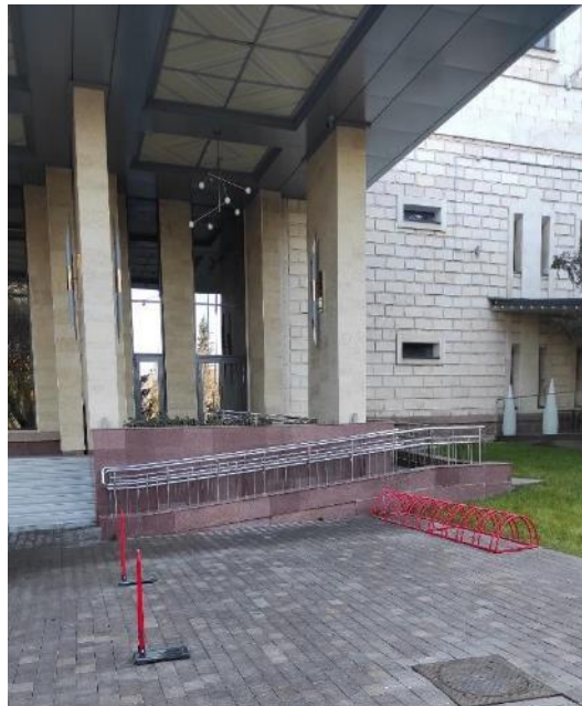
Photo 4. Proper installation of the ramp for persons living with disabilities in Hotel B in Almaty, Kazakhstan. 16
